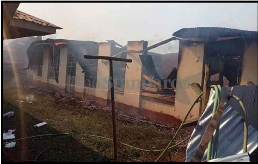
Figure 1.1: Dormitories of Kisumu High School damaged by fire in August 2022 (The Standard, 2022)
