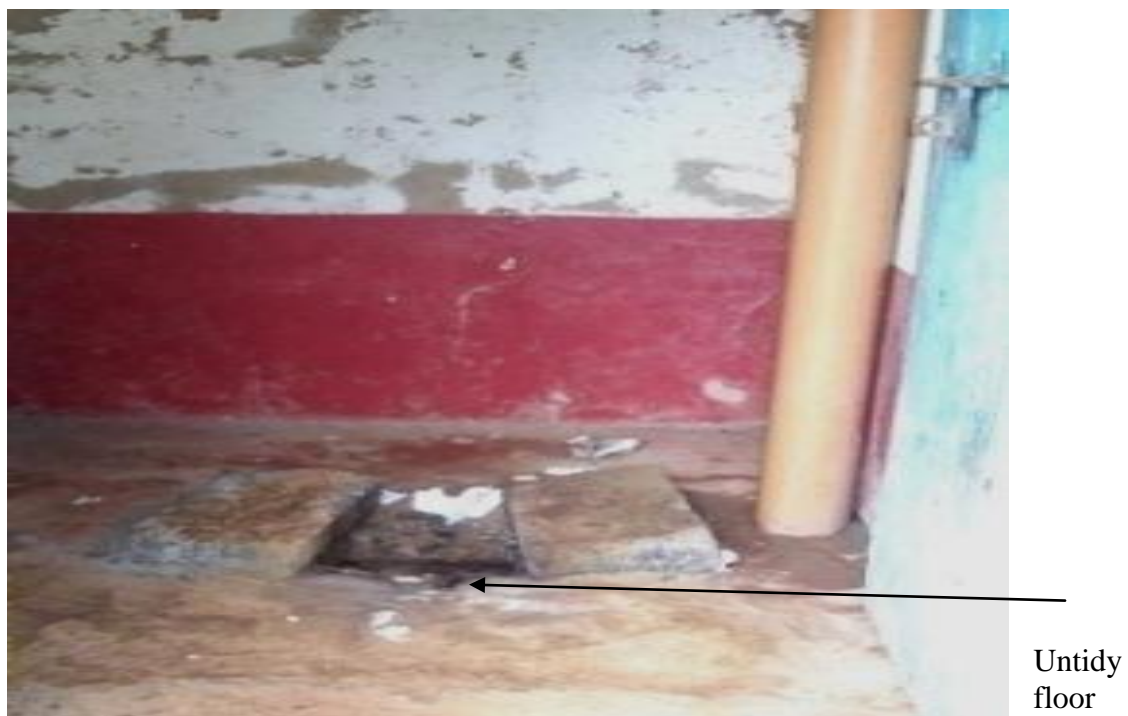
Plate X: Concrete Pit Latrine with Untidy floor at Kona Mbaya (Source: Author, 2011)
