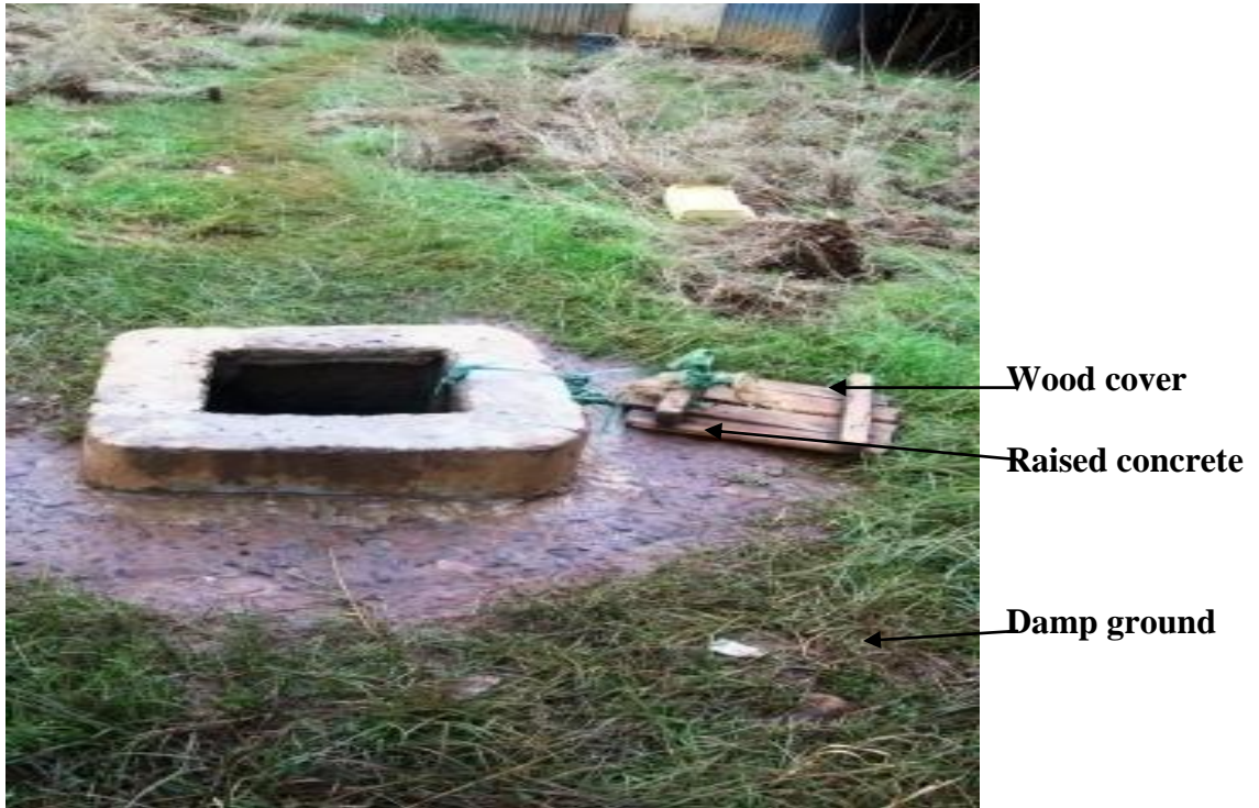
Plate S: Concrete Raised Wood Covered Borehole at Kambi Nguruwe (Source: Author, 2011)
