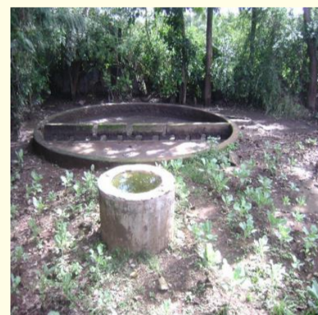
Fig. 5. Failed and abandoned digester at Kirinyanga county
