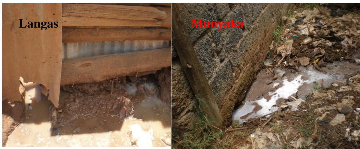
Figures 4.10: Human waste being released to the environment from toilets in Langas and Munyaka (Source: Author, 2013)
