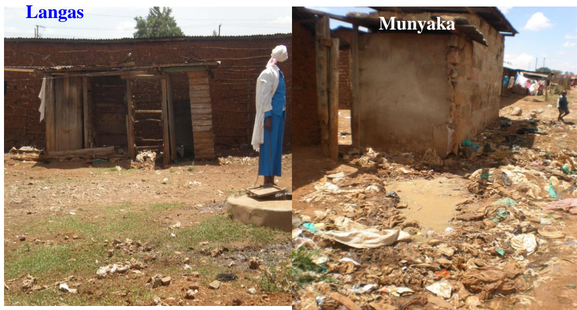
Figure 4.1: Pictures showing a dilapidated pit-latrines
