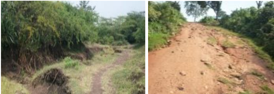
Plate 4. 3: Roads eroded by water in lower and upper Oroba water catchment (Source: Author, 2012).
