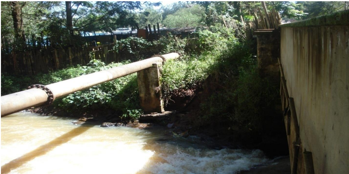
Plate 14: Encroachment of structures on River Sosiani's Riparian Reserve. Source: Field Data
