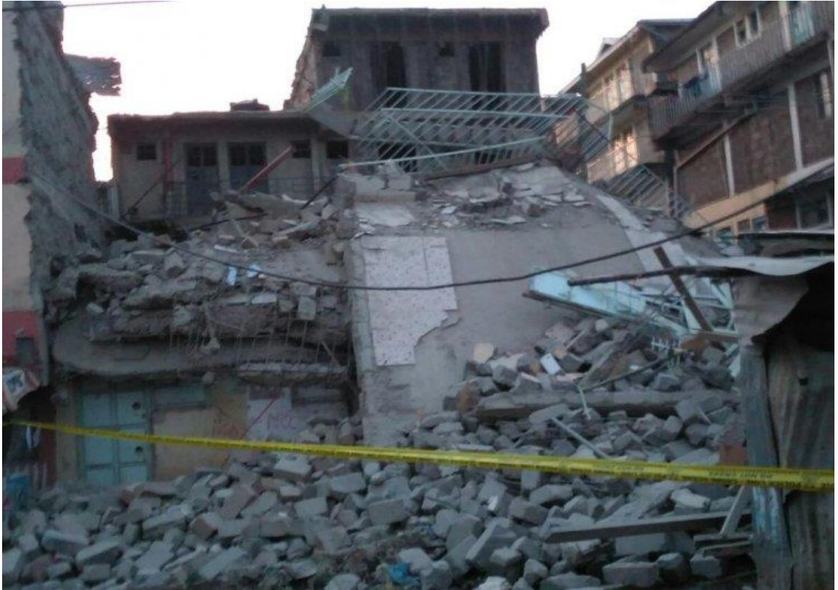
Figure 2.7 Shows a Four-Storey building which collapsed in Zimmerman area in Nairobi on 9th March 2016. Source: http://www.the-star.co.ke/news/27/3/2016;11:00 hrs
