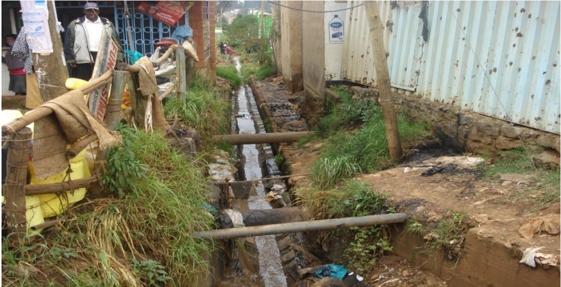
Plate 3: Construction of structures on top of water and sewer lines in the CBD. Source Field Data
