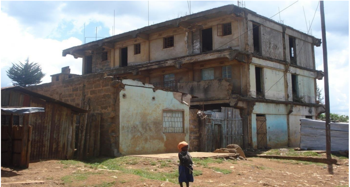
Plate 11: Demolished part of the building that encroached on the Road Reserve along Yamumbi - Langas Area. Source: Field Data
