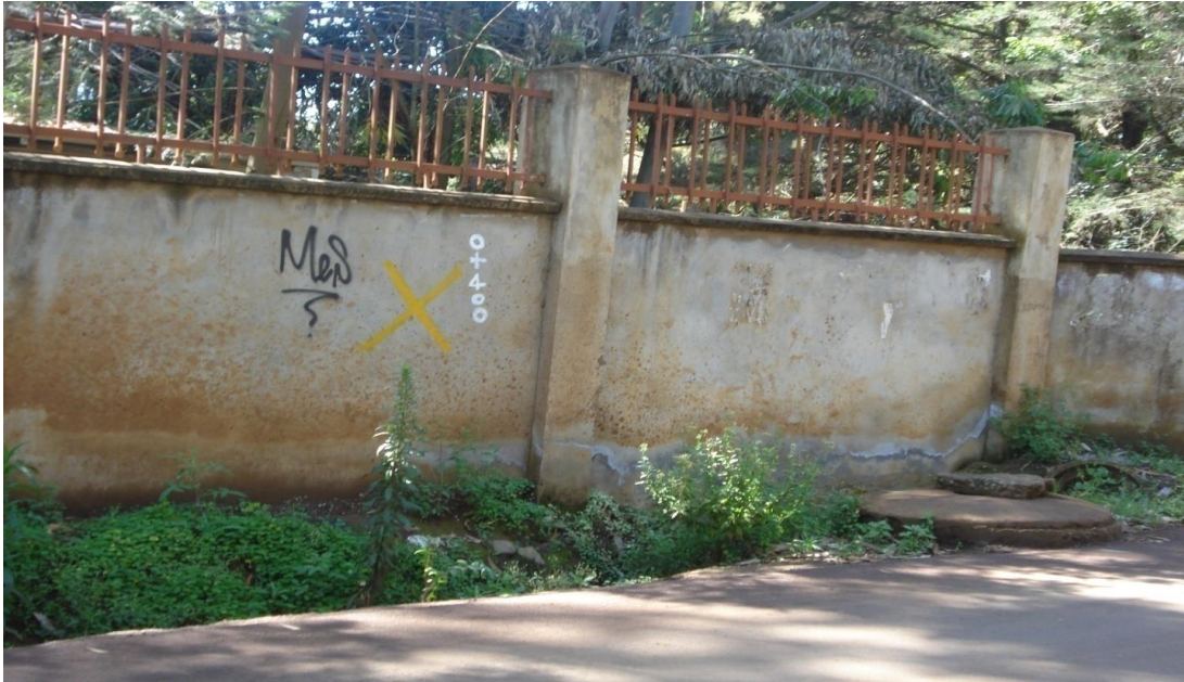
Plate 13: Encroachment of the roads by structures at Elgon View Road. Notice KURA's Yellow X Marking. Source: Field Data
